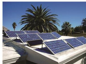
Solar PV System
